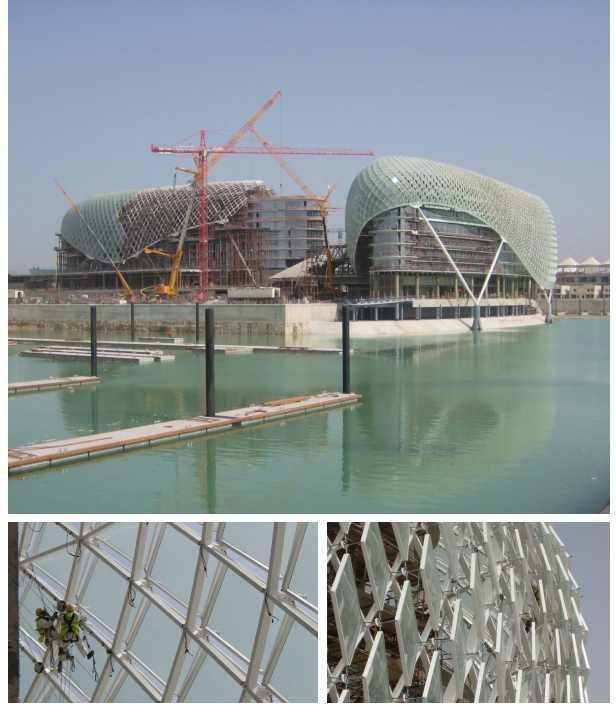
Figure 4: Yas Island Hotel during construction. At bottom left one can see a detail of the outer skin which exhibits torsion-free nodes (images courtesy Waagner-Biro Stahlbau).
