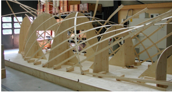
Figure 2: Assembling screw-laminated beams for a timber rib shell prototype based on a 2-pattern of geodesics supported by a third family of vertical elements [PW06]. This is no web. Image courtesy IBOIS (EPFL, Lausanne).
